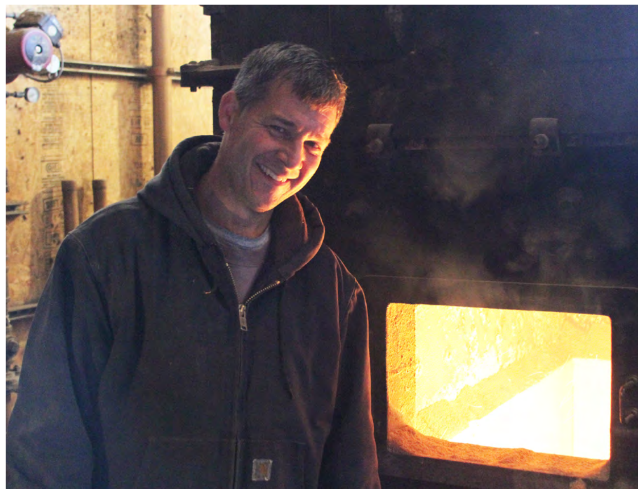
Brad Cox with the Dry Creek Community biomass boiler.
