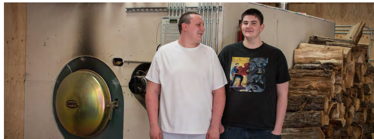
Student boiler operators at the Prince of Wales School.
